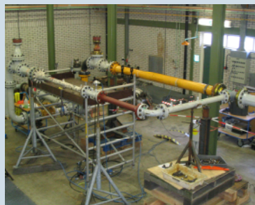
KEMA test facility, Groningen, the Netherlands
