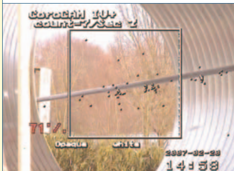
▲ Corona discharges, as photographed using the UV camera.
