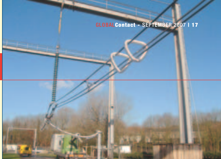
▲ The complete test rig, with the conductors, the corona shields, the spacer, the insulators and the test transformer. The latter is used to vary the voltage so the investigators can determine the electrical field at which most discharges occur.
